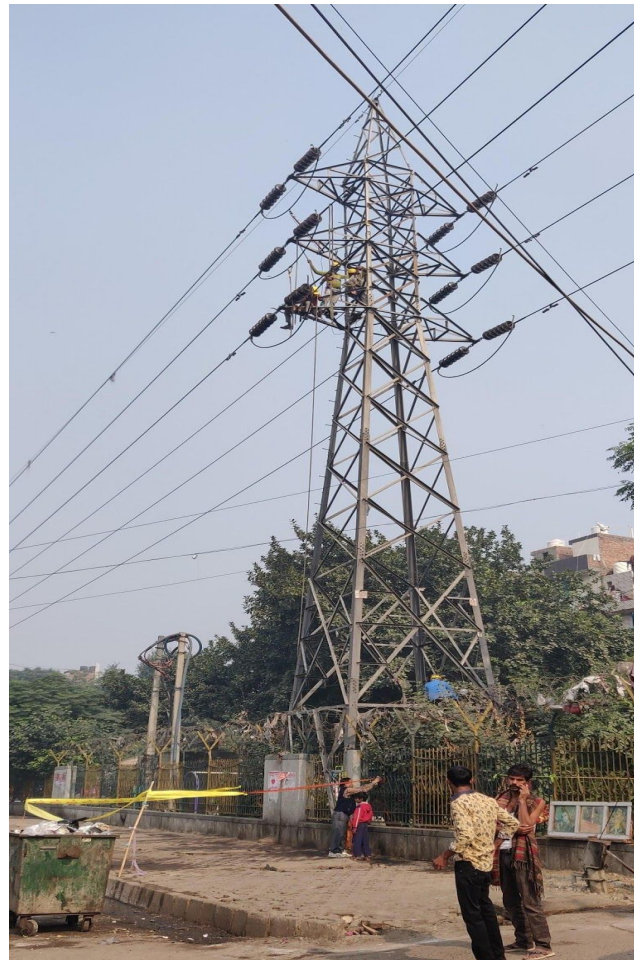
In picture: Workers repairing the wiring system so that outages can be reduced
